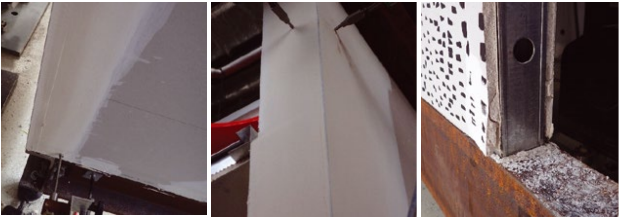
■ PHOTOS 3,4 & 5 – R2 L/360 (±5.40MM) EXTERNAL CORNER, NIB WALL END, DOOR OPENING BASE DAMAGE
