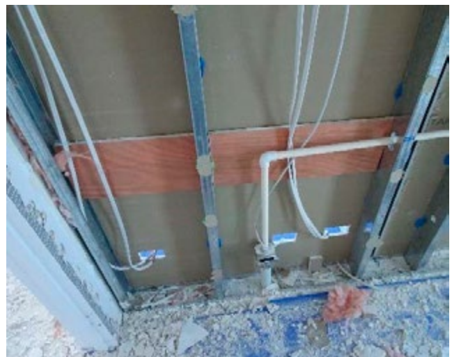
■ MISSING GROMMET AND PIPE SCRAPING ON STUD WEB CAUSING NOISE
